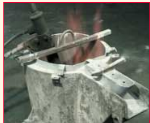
Figure 3: The KALTEK ISO reaction being initiated with a gas burner
