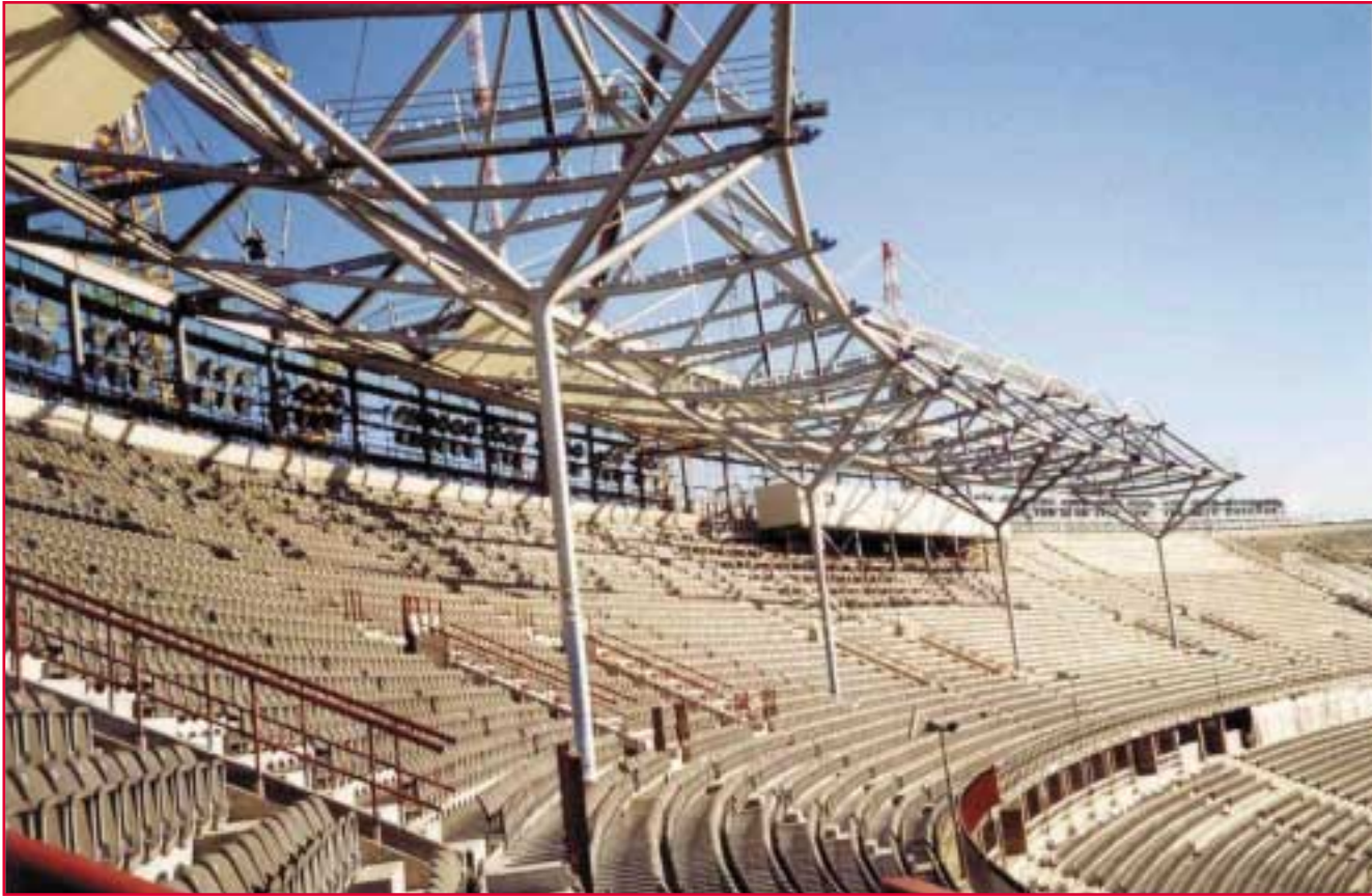
Figure 2: Initial roof construction. Architects: von Gerken, Mang and Partner. Photo: Heiner Leiska
