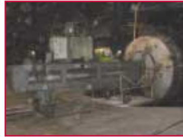
Figure 5: Lining extraction using a jack actuated with a maximum pressure between 120 and 300bar
